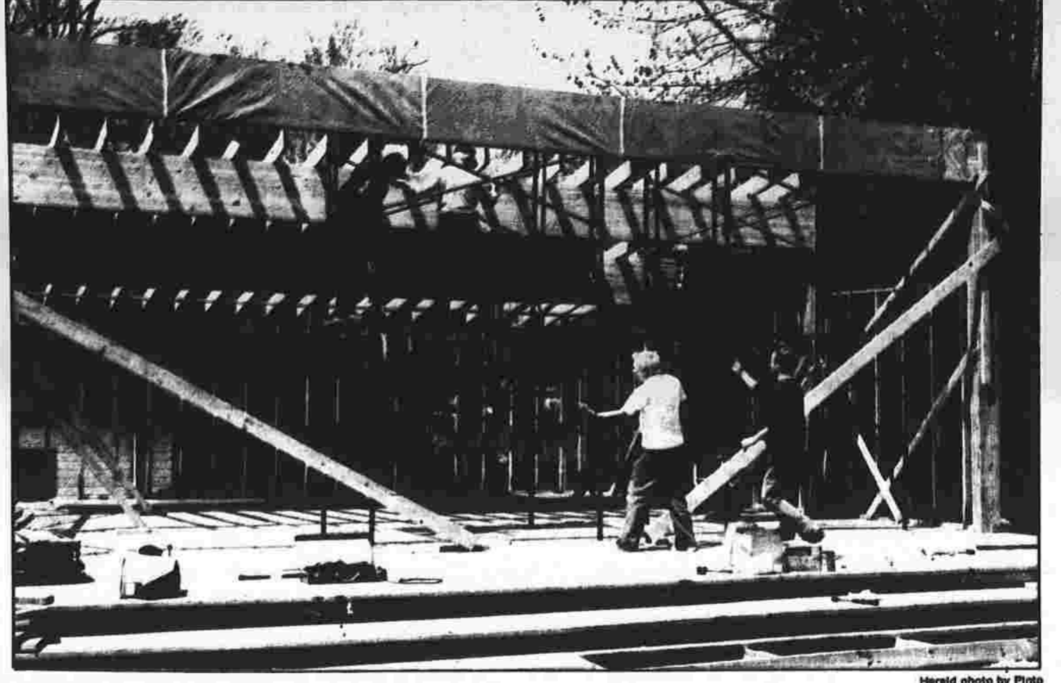
Members of the Coventry Lions Club work on the new band shell at Patriot's Park in Coventry. The facility will not be completed in time for dedication by Memorial Day, the club says, although it will be ready for the town's 275th anniversary celebration in July.
